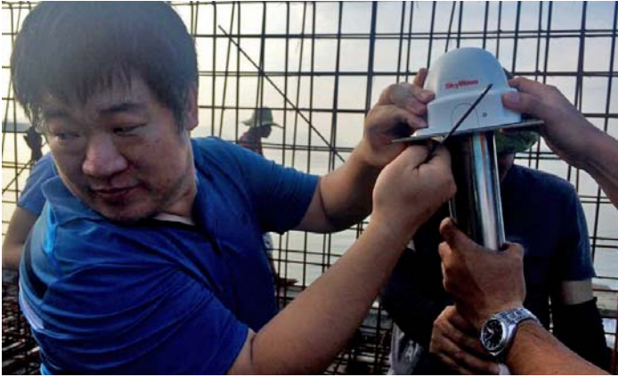
Mr. Deokwan Choi of KHOA installing the satellite communications antenna for the tide gauge instrument
