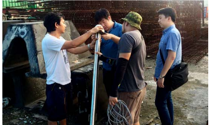
Installation of Automatic Weather Station of Tacloban Tide Station with NAMRIA personnel Ellison Parojinog (left) and three KHOA personnel
